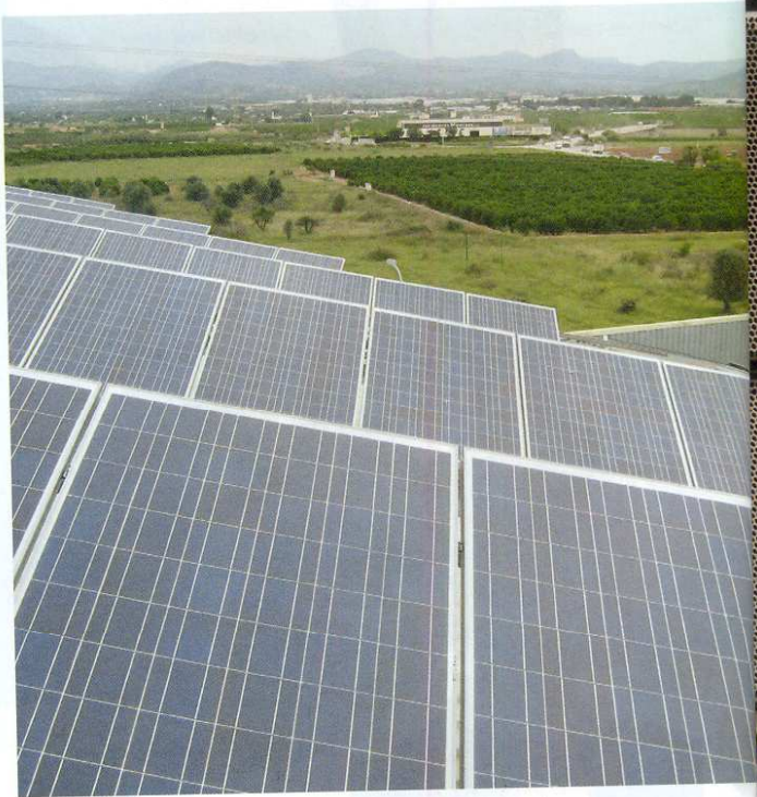
Solar panels grace Beyma's Spanish facility
